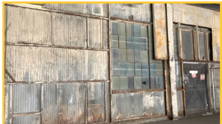
The 1940s-era warehouse structures are not adaptable to support NAVWAR's mission requirements.
